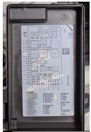
D. Relay Panel Inside Cover
